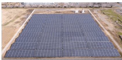
Solar power panels installed by Mie Works (started operation in April 2021)
