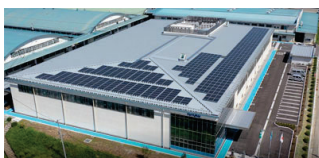
Solar power panels installed by TOTOKU Electric Co., Ltd. (started operation in January 2021)
