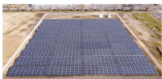
Solar power panels installed by Furukawa Automotive Systems Inc. headquarters (started operation in January 2022)
