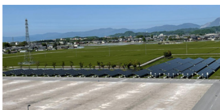
Solar power panels installed in Furukawa Automotive Systems Inc. headquarters (started operation in January 2022)
