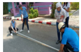
Repainting white lines on roads and playgrounds in local elementary schools in 2023 (FAST*)
