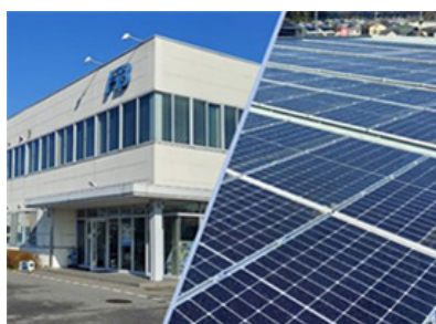
Solar power panels installed in The Furukawa Battery Co., Ltd. (started operation in April 2022)
