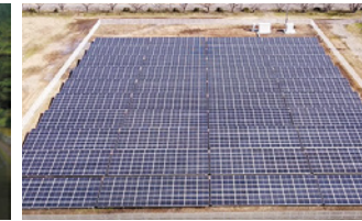
Solar power generation panels installed by the Mie Works (operation start, April 2021)
