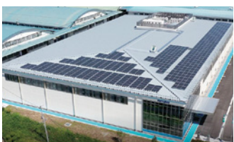
Solar power generation panels installed by Totoku Electric Co. (operation start, January 2021)
