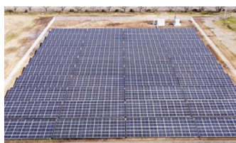
Solar power generation panels installed by the Mie Works (operation start, April 2021)
