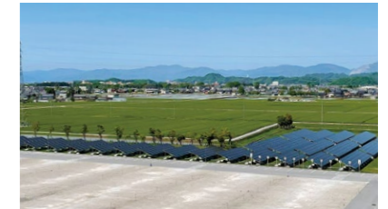
Solar power generation panels installed at the Headquarters of Furukawa Automotive Systems Inc. (operation start, January 2022)
