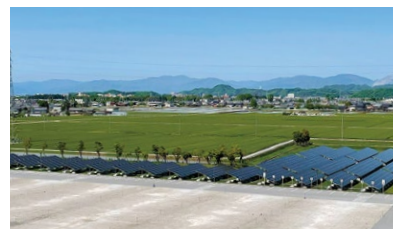
Solar power generation panels installed at the Headquarters of Furukawa Automotive Systems Inc. (operation start, January 2022)
